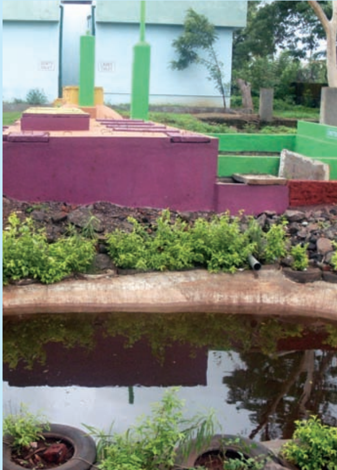
Decentralised wastewater treatment system at Adarsh Vidyalaya, Kulgaoon Badlapur Distt Thane.
