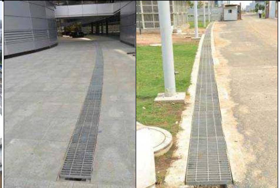
Surface & Road Rain water collection
