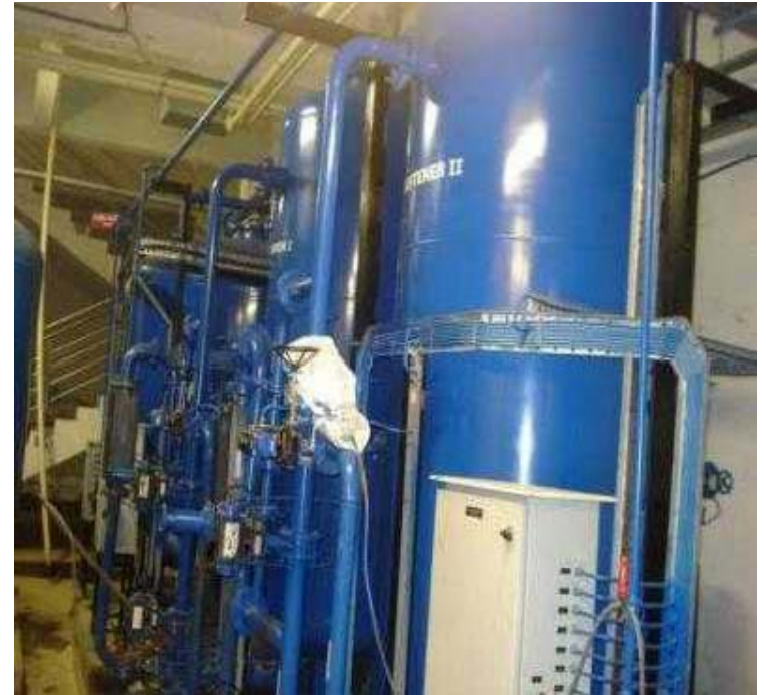
Treatment plant for pond water
