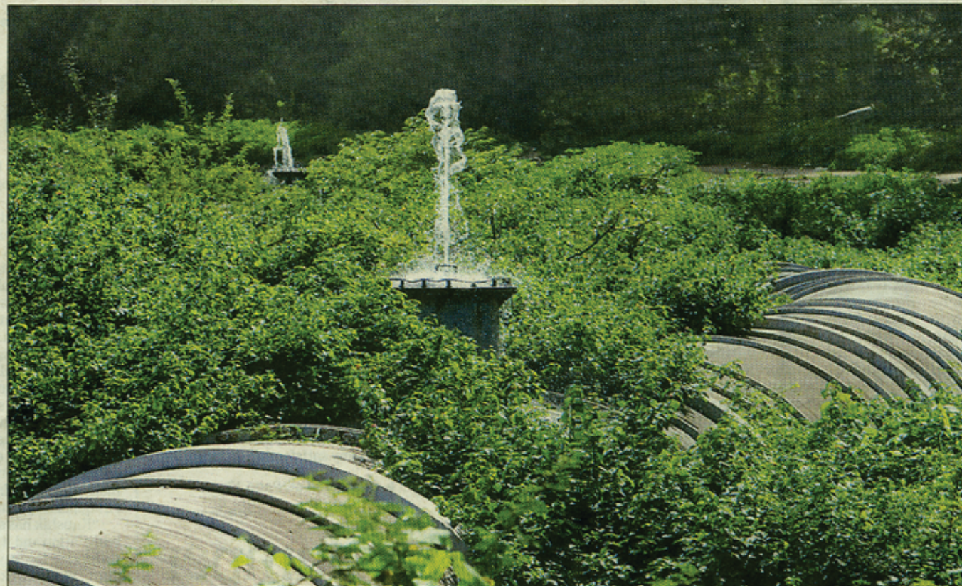
The pipeline carrying water to the city often springs leaks leading to wastage of water
