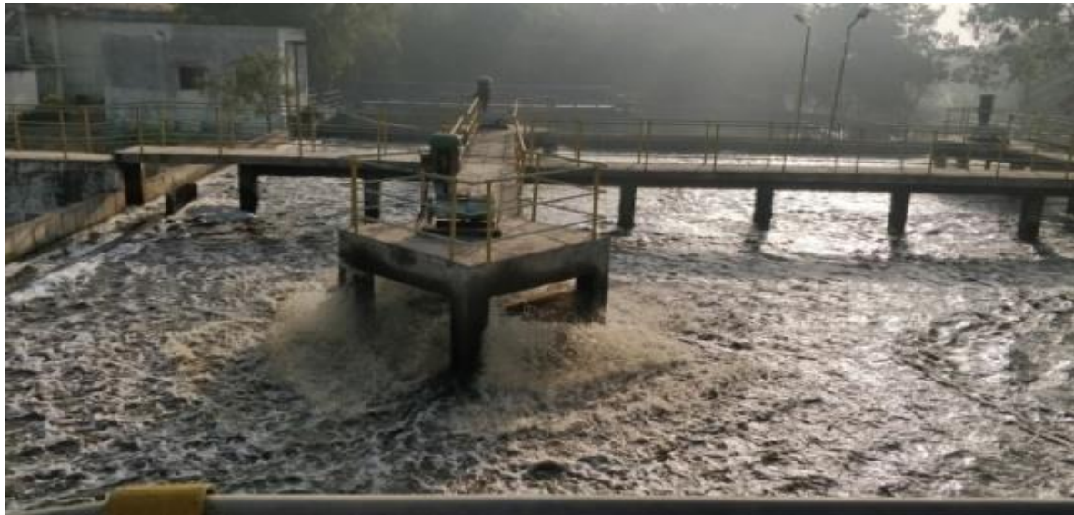
Figure 2: Sewage Treatment Plant of 130 MLD capacity, Tapovan, Nashik (Source: Mudit/CSE, 2020)
