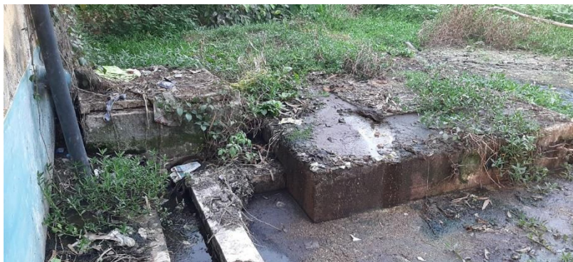
Figure 3: Septic tank connected to open drain, Source: Manish/CSE, 2020
