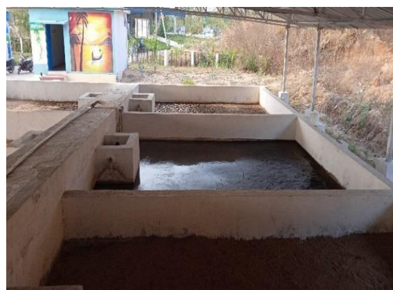
Figure 7: Sludge drying bed in FSTP (Source: Vandana/CSE, 2020)
