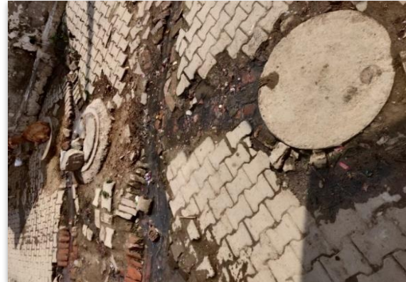
Choked sewer line
