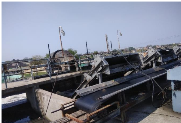
Inlet of Bingawan STP
