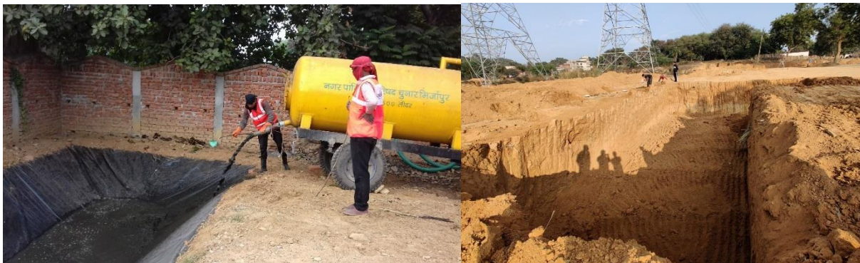
Figure 4: Temporary trenching facility (on the left) and Faecal Sludge Treatment Plant (on the right) (Manish/CSE, 2020)
