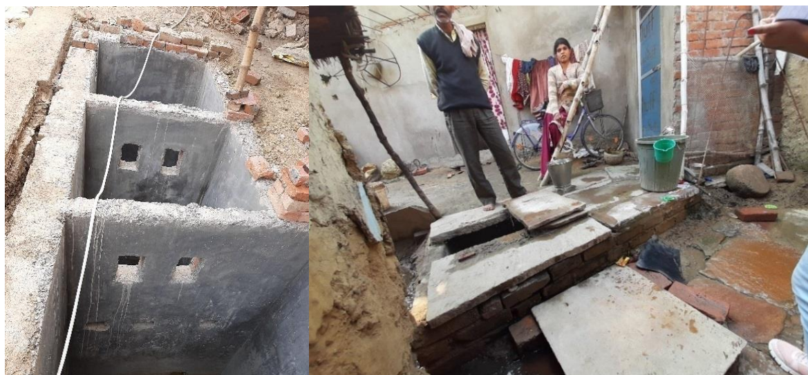
Figure 2: Septic Tank under construction and fully lined tank connected to open drain (Manish/CSE,2020)
