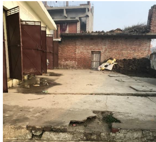
Figure 4: Septic Tank of a Community Toilet at Harijan Basti (Harsh/CSE, 2020)
