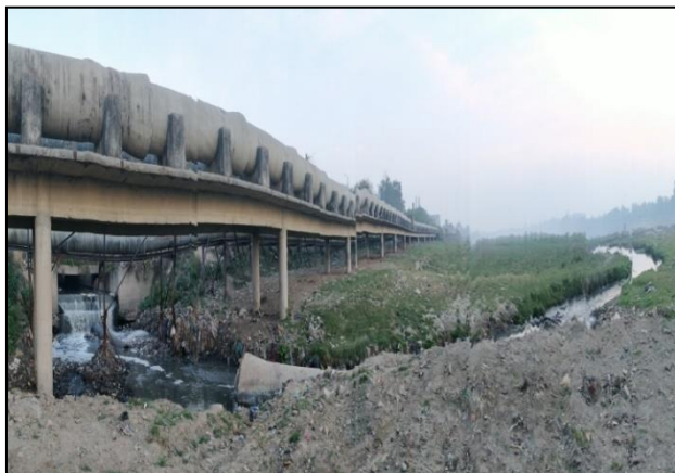
Figure 4: Storm water drain directly discharging into Yamuna river
