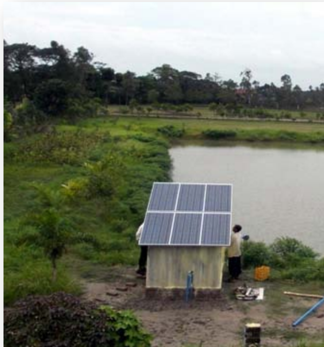
Micro Solar Pump House
