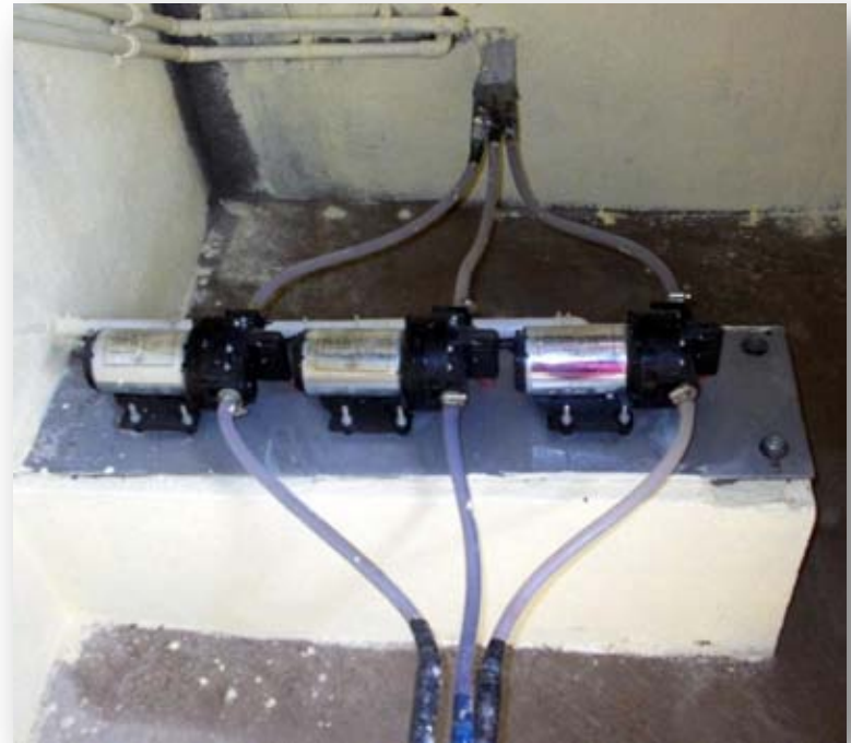
Micro Solar Pump under operation
