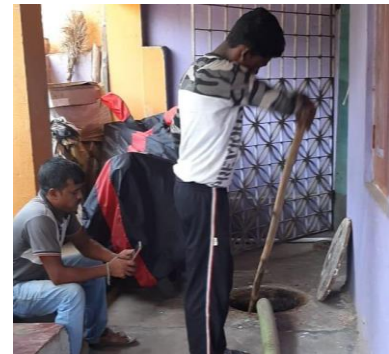
Figure 5: Emptying Onsite Sanitation System by Vacuum Tanker (Source: CSE,2020)
