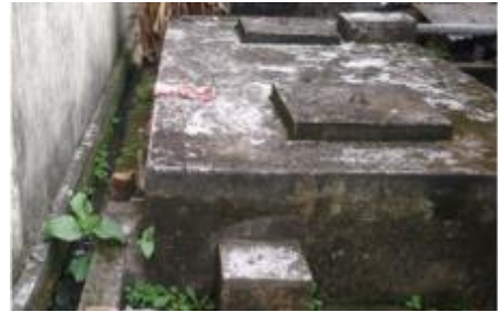
Figure 3: Septic Tank (3-chambered) in Ward no. 9
