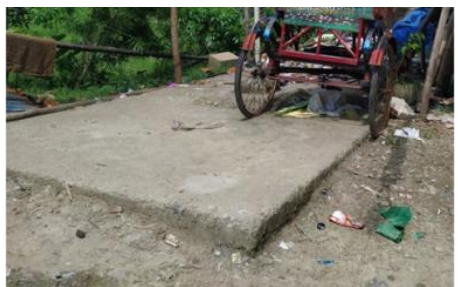
Figure 4: Septic Tank (3-chambered) in Ward no. 13 (Vikash/CSE/2020)
