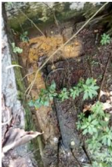
Figure 2: Night Soil discharged directly into open drains
