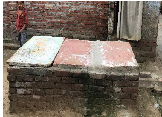
Figure 4: A fully lined tank connected to open drain. (Harsh/CSE/2020)
