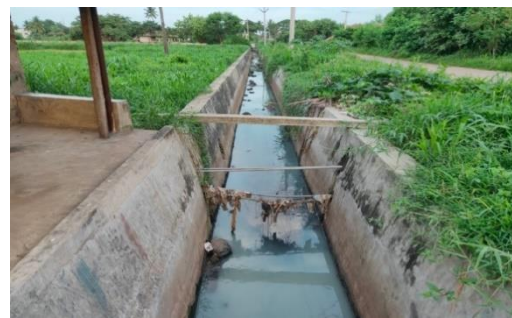
Figure 4 : Wastewater & supernatant flowing in storm water drain
