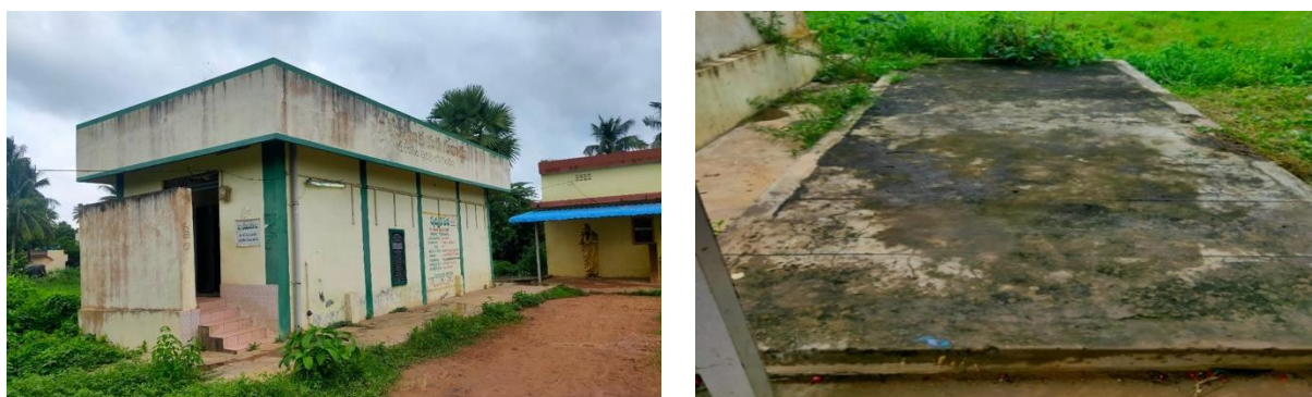
Figure 2: Community toilet (left) and Septic tank in community toilet (Right)
