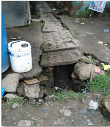
Figure 1: Open drains carrying wastewater in Kabutar Khana
