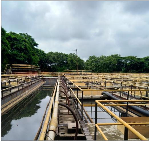
Figure 3: STP of 78 MLD capacity with UASB technology
