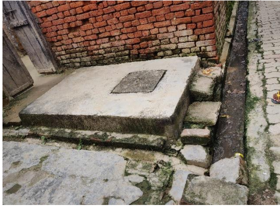
Figure 1: Overflowing containment system (Nida, CSE, 2020)
