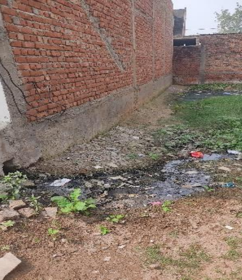
Wastewater collecting in empty plots-ward 7
