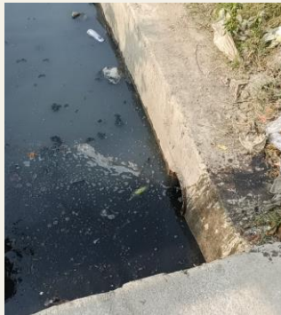
High presence of blackwater in drain in ward 17
