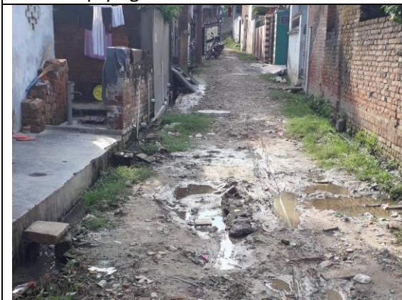
Phaphamau (Nagar Nigam Area not in Study Area) – sewer lines laid in narrow lanes
