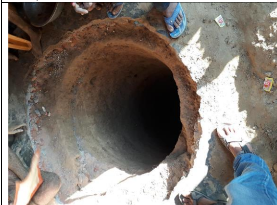
Containment under construction in Karehada Village near Numayadahi STP (In Study Area). More than 25 feet deep. Emptying frequency more than 15 years
