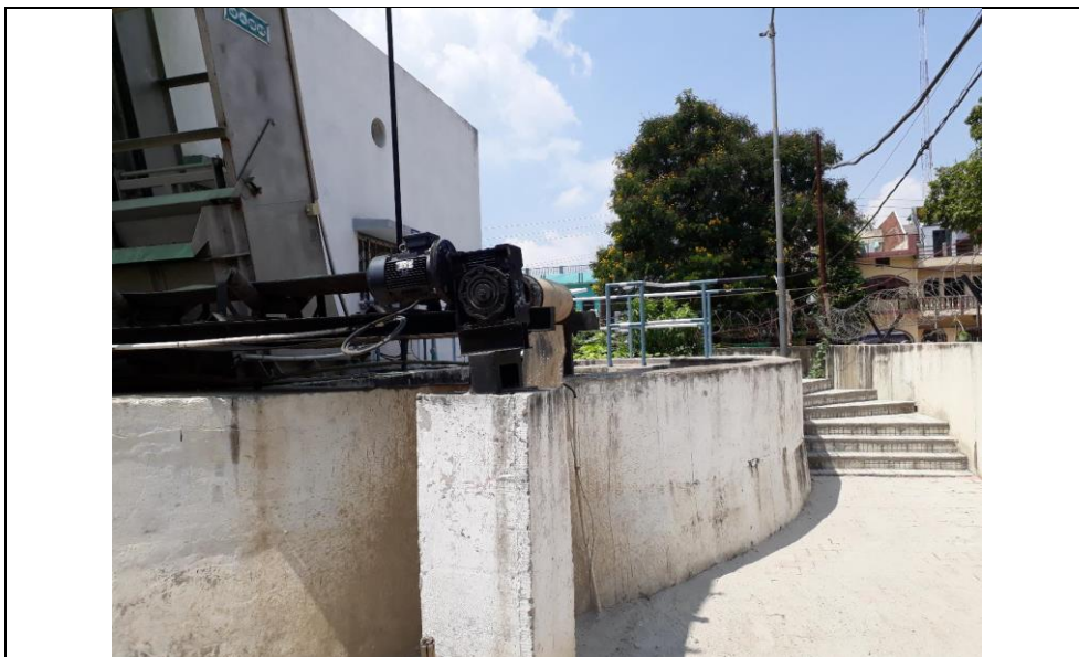
A Receiving Unit near the SPS Sump can be proposed for Co-Treatment
