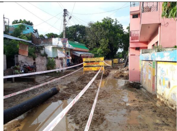
Phaphamau (Nagar Nigam Area not in Study Area) – Sewer lines being laid
