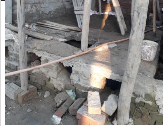
Saha Urf Pipalgaon (Village in Study Area) – septic tank under construction which would need emptying
