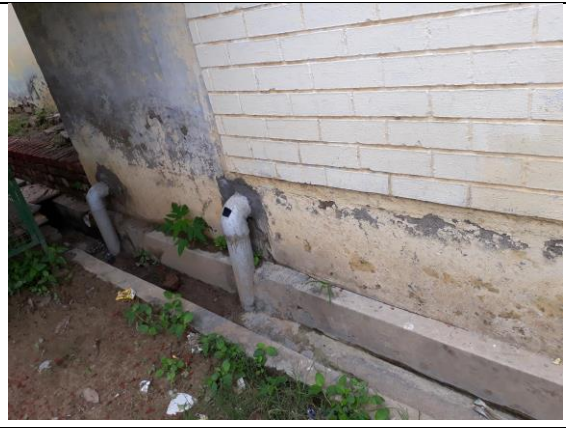
Septic Tank outlet connected to sewerage system
