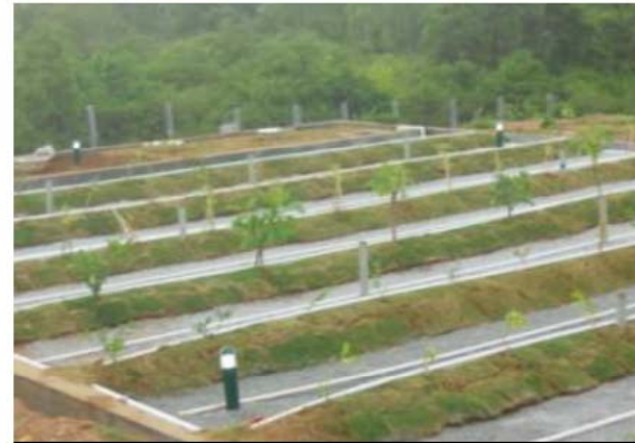
75 KLD plant at FRLHT Hospital, Bengaluru
