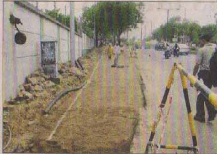
The revised road boundary being marked out adjacent to the ISRO wall on the Jodhpur Ramdevnagar stretch
