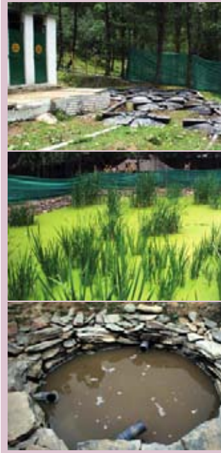
Cleaning the waste of millions: toilets are dosed with microbes and so don't smell, waste goes to a reed bed and oxidation tank.
