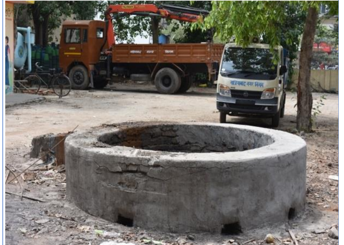
Decanting Station at Mohan Nagar SPS
